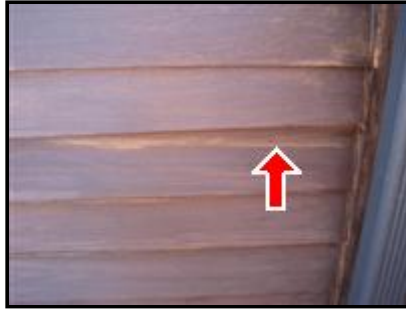
C. Picture 1 Loose siding piece - top level near west side
