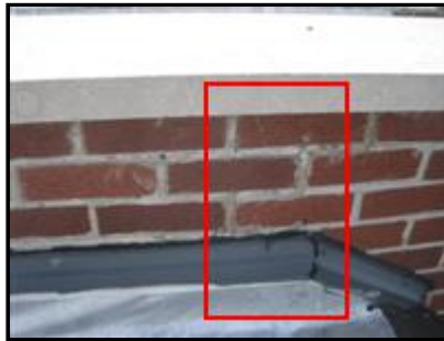
L. Picture 4 Cracked bricks - east wall
