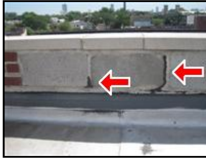
L. Picture 2 Caulk on cracks
