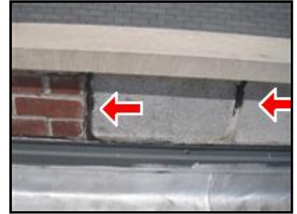
L. Picture 3 Caulk on cracks
